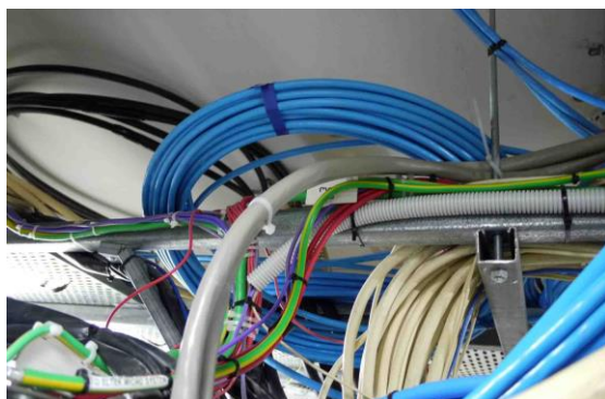
Figure 3: Incorrect cabling above MDF
